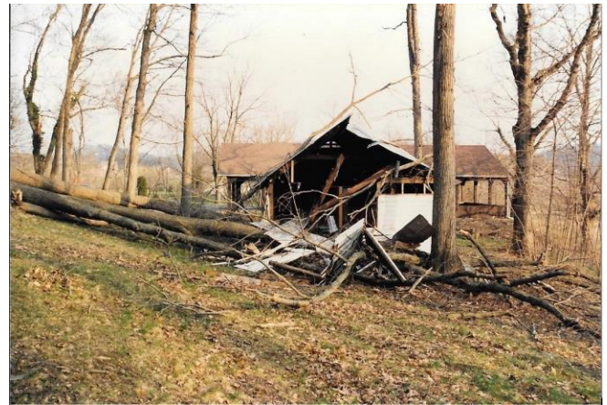
Refreshment stand damaged by fallen tree, April 1993
